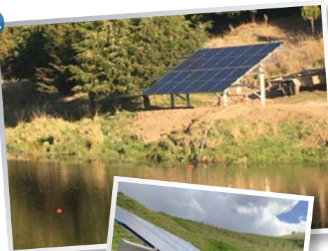
14-15 Hawkes Bay Area: 12 Panel Solar Project, 5.7kW's of Solar Power, 20m 3 per day at 150 mtrs, head Helical Rotor Submersible Pump, Pump suspended on Dam Pontoon
